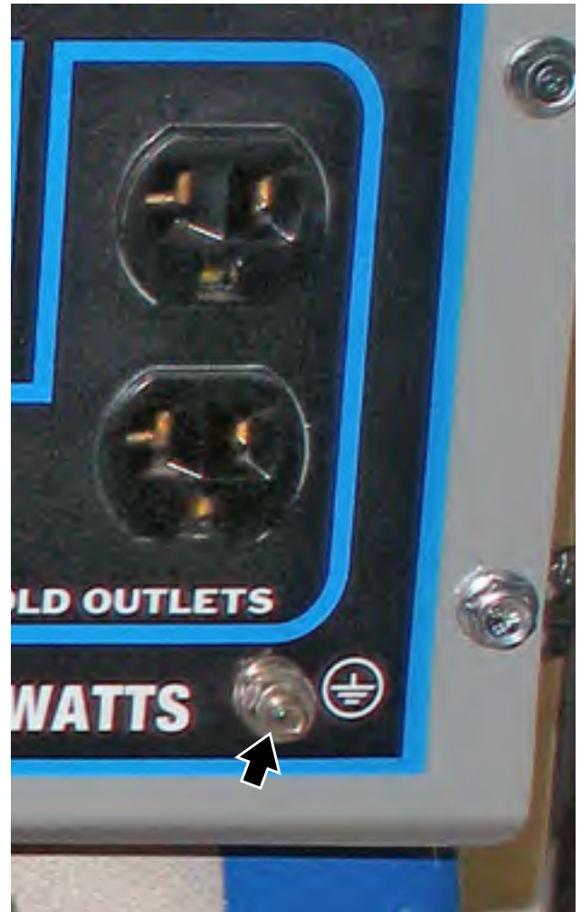
Figure 12 – Ground Terminal on the Control Panel
